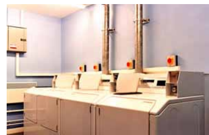
Laundry room at Sebastian Street
