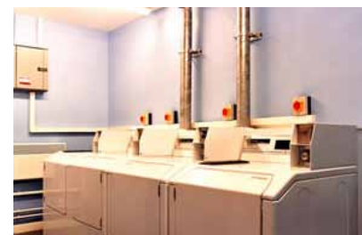
Laundry room at Sebastian Street
